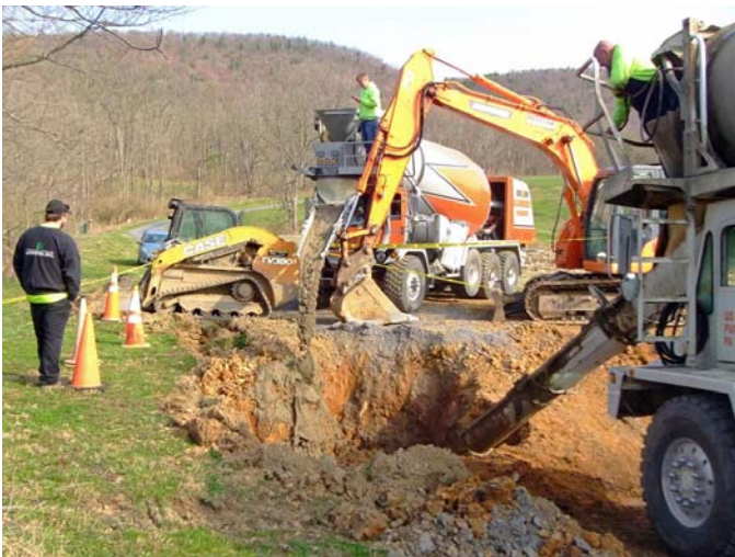
Three mixer truck loads of cement flowable fill go into the excavated sinkhole. D. Glick photo
